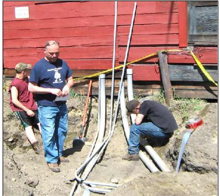
Vocational Technical School would-be electricians installing underground wiring as part of site preparation for the carbarn project.
