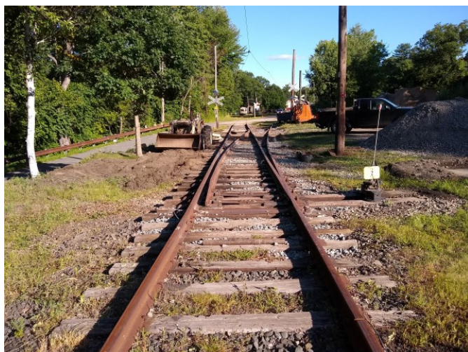
Looking towards the Car Barn at the rebuilt turnout 2, where the House Track splits from the Main Track
