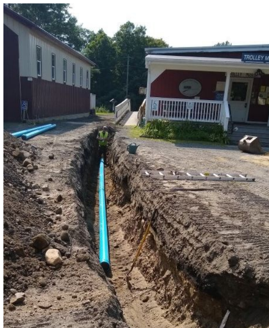
This new 6" water main from Elm St to the Freight House will allow us to eventually add fire protection to all our buildings.
