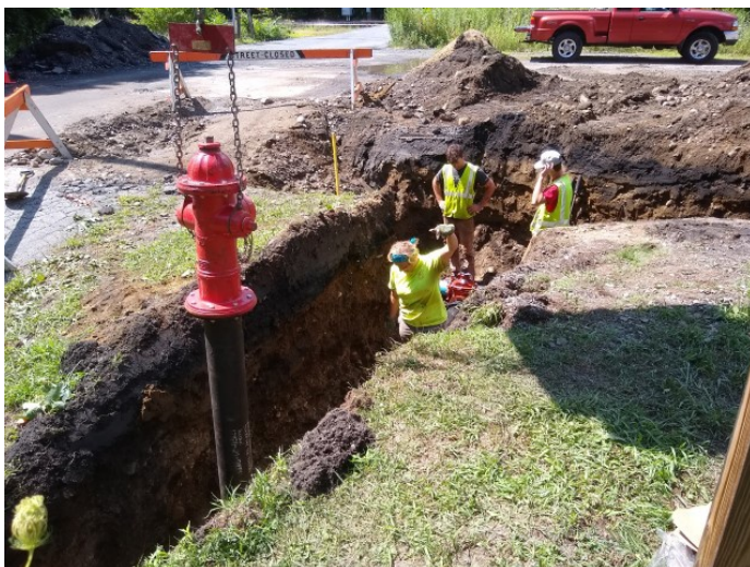
The Shelburne Falls Water Department crew guide our new hydrant into place
